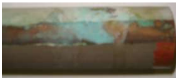
Figure 1. Copper corroded tube.
