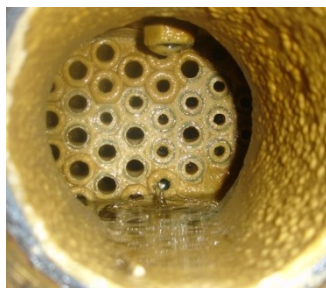
Figure 1. Amorphous silica deposits on industrial equipment.
